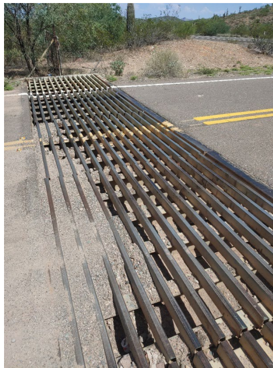
Figure 63. Crossing Guard with More Than 50 Percent Sedimentation
