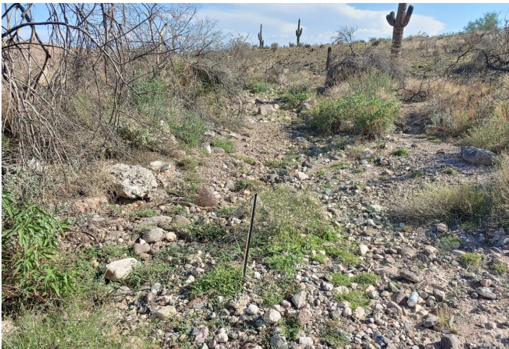
Figure 58. ROW Fence Blowout Across a Wash Caused by a Flood
