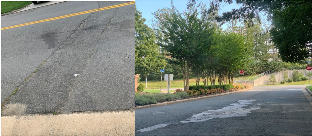
Figure 6-26. Two roads with patching labels.
