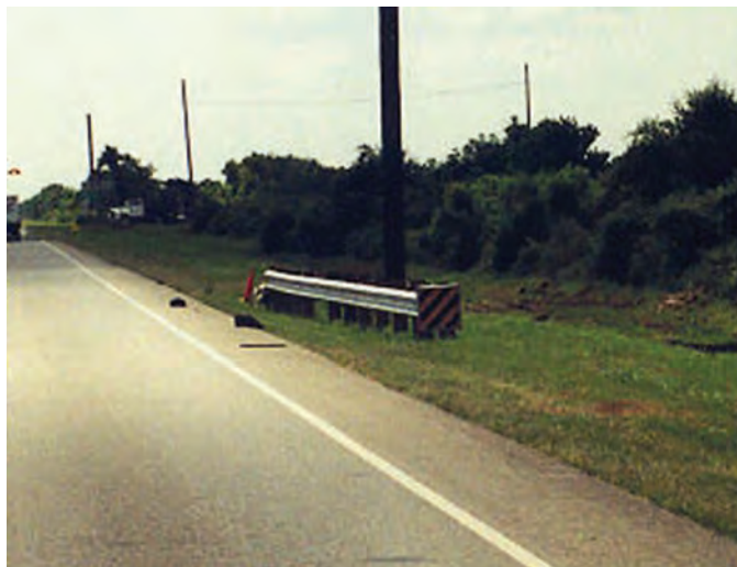
Figure 25. Example of guardrail and extruder terminal (Photo: Don Ivey).
