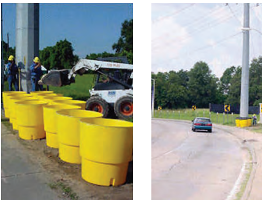
Figure 22. Examples of installations of sand barrel crash cushions (Photos: Don Ivey).
