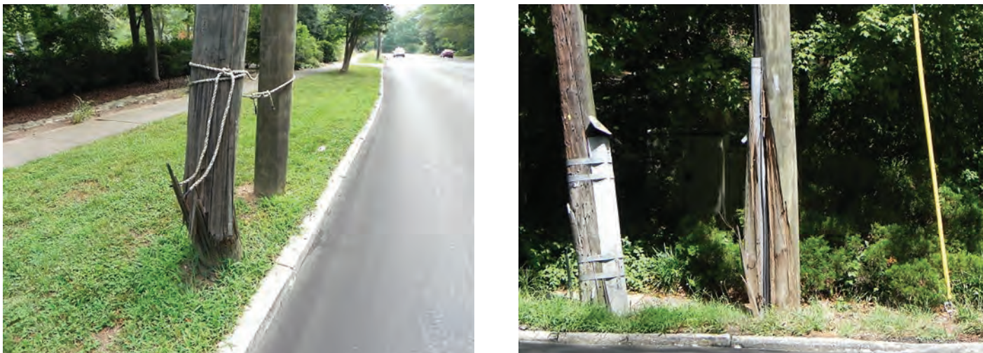
Figure 14. Examples of damaged high-risk poles (Photos: Kevin Zegeer).
