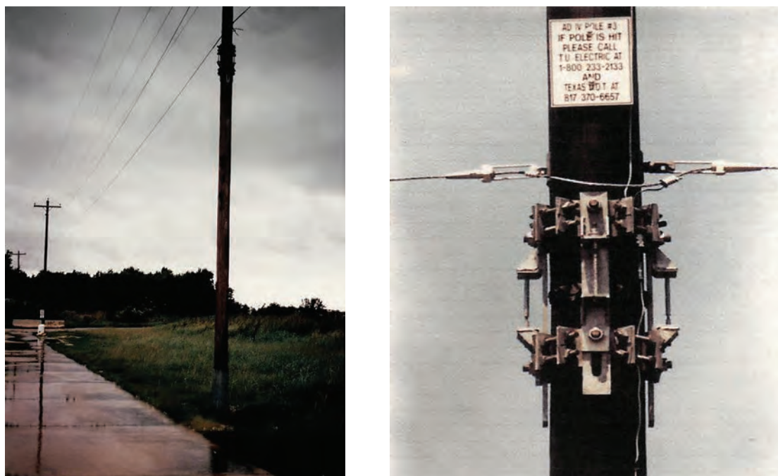
Figure 24. Examples of steel-reinforced safety poles (Photos: Don Ivey).
