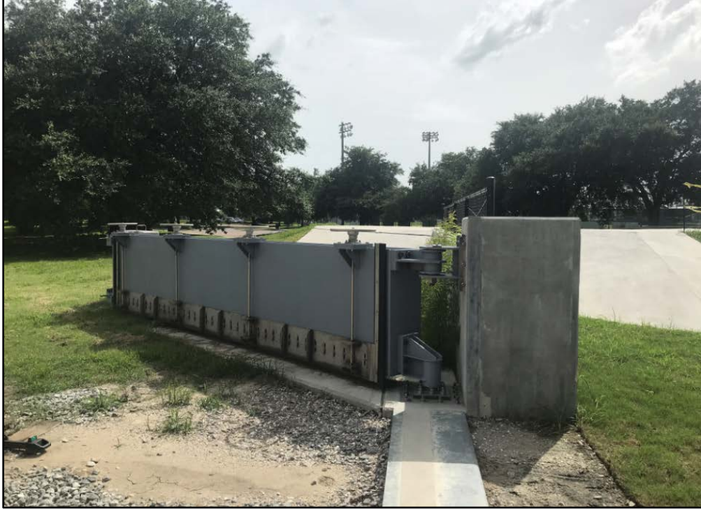
Figure 3-18: Single-leaf Swing Gate in New Orleans at a Railroad Crossing (M&N)
