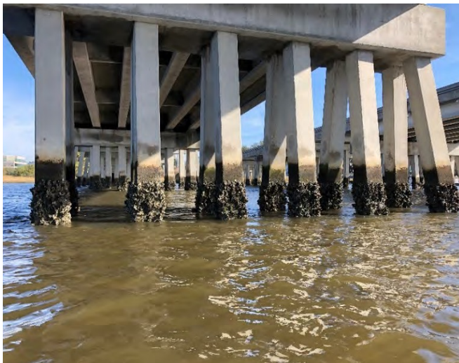
Oysters on existing bridge structures in the Ashley River. (Photo by Three Oaks Engineering)
