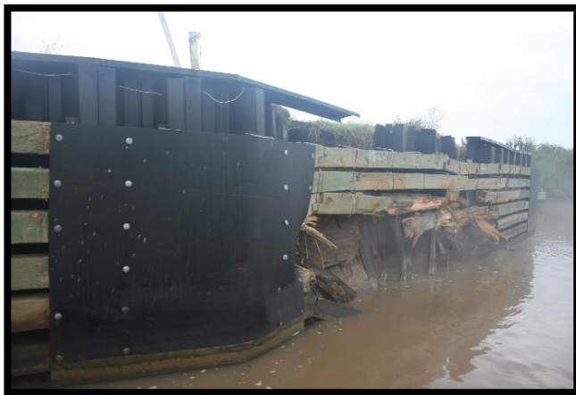
Figure 3-2 – Guidewall Damage from Barge
