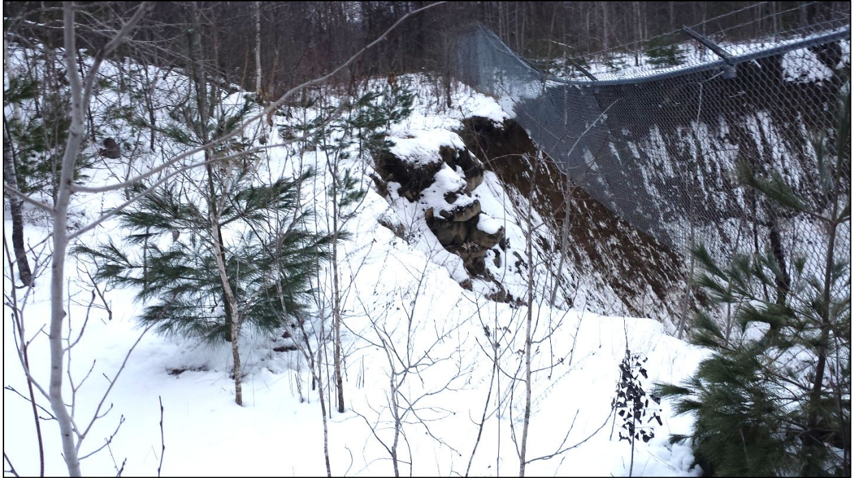
Figure 3-2. Subsiding mine shaft seal at Joker Shaft, December 8, 2016 (Source: staff).
