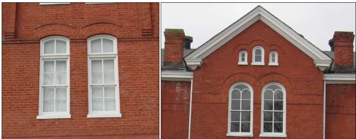
FIGURE 3-215: FIRST STORY WINDOW DETAIL, EAST ELEVATION (LEFT); SECOND STORY AND GABLED WINDOW DETAIL, EAST ELEVATION (RIGHT)
