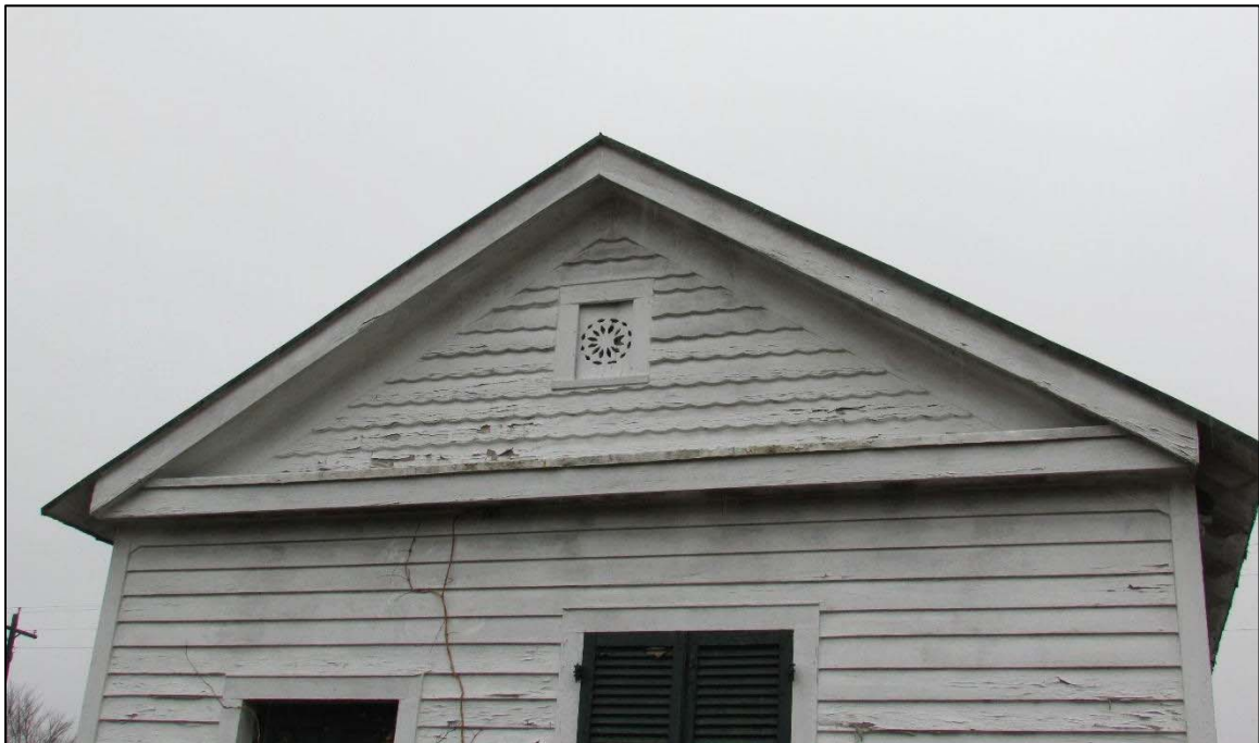
FIGURE 3-71: FIRST WOODFORD POST OFFICE, DETAIL OF SCALLOPED SIDING AND DECORATIVE VENT IN GABLE OF FAÇADE
