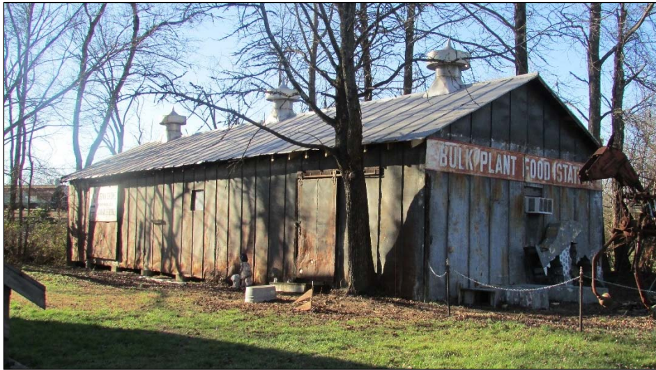
FIGURE 3-173: FRAME OUTBUILDING, SOUTHEAST OBLIQUE. PHOTO FROM THE FEBRUARY 2016 RECONNAISSANCE-LEVEL SURVEY OF THE DC2RVA PROJECT.
