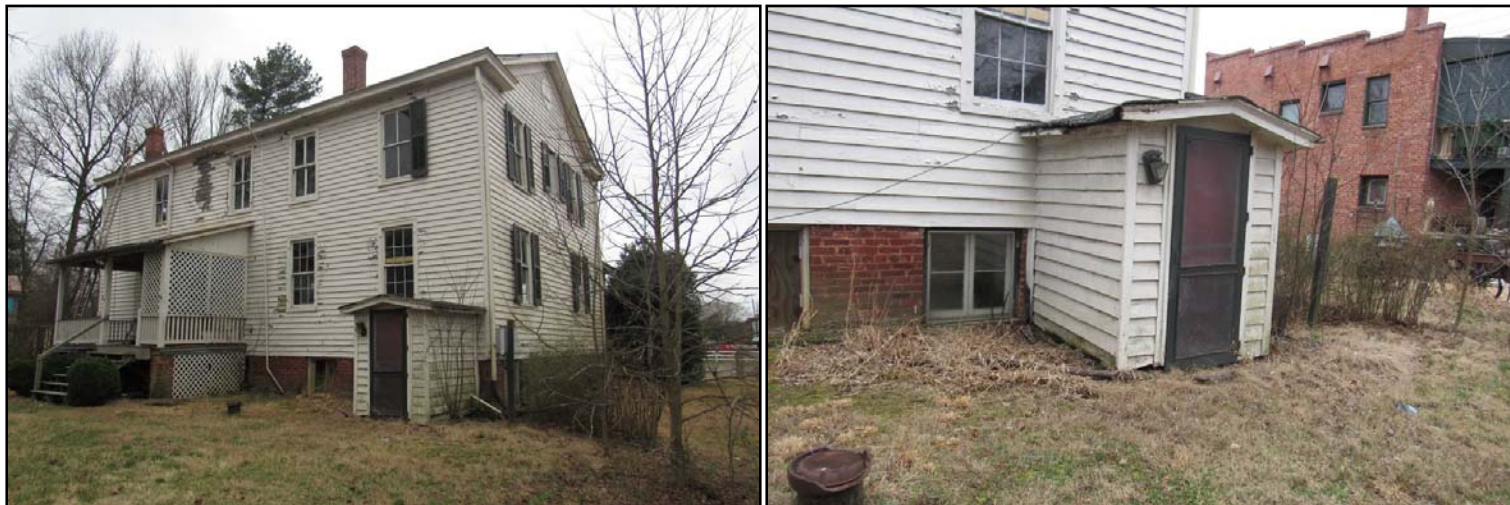
FIGURE 3-186: NORTHEAST OBLIQUE (LEFT); CELLAR ENTRANCE ON NORTH SIDE OF EAST ELEVATION (RIGHT)
