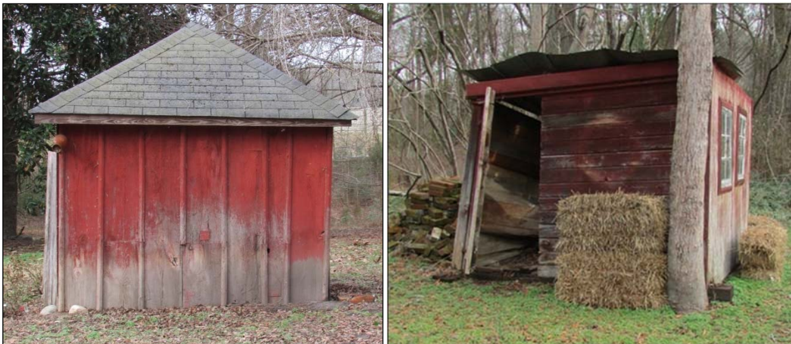
FIGURE 3-150: SOUTH ELEVATION OF CIRCA-1911 SHED (LEFT); NORTHWEST OBLIQUE OF CIRCA-1925 SHED (RIGHT)
