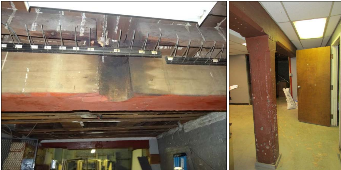
FIGURE 3-18: EVIDENCE OF MILL SHAFT IN WESTERN STORAGE AREA OF BASEMENT, FACING SOUTH (LEFT); BASEMENT, FACING WEST (RIGHT)
