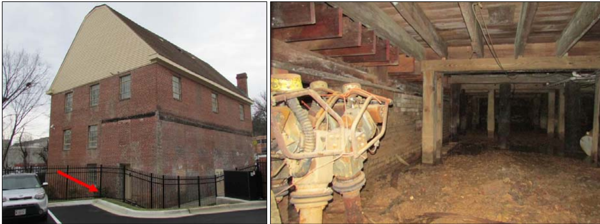
FIGURE 3-19: SUBBASEMENT ENTRANCE (DENOTED BY RED ARROW), SOUTHEAST OBLIQUE (LEFT); VIEW OF SUBBASEMENT, FACING NORTH (RIGHT)
