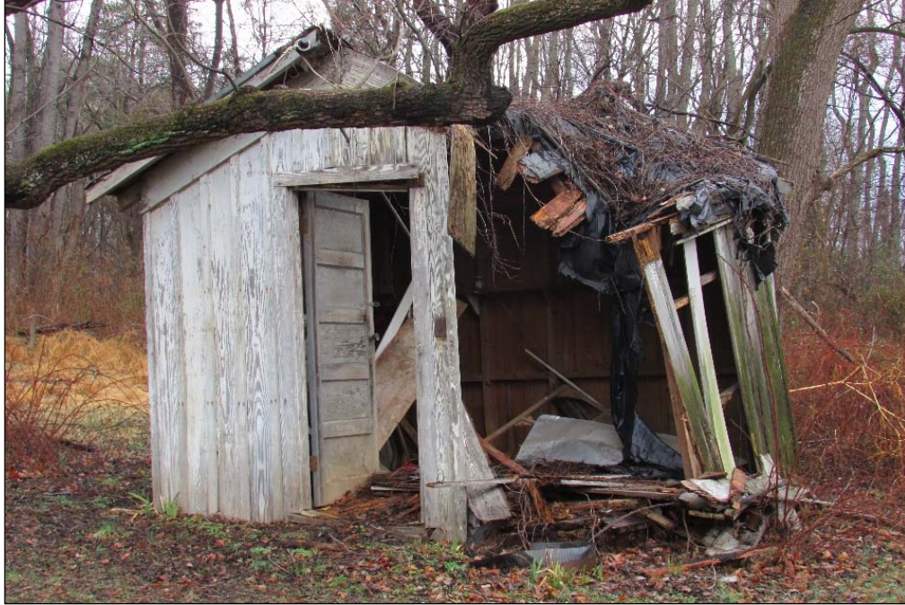
FIGURE 3-31: SOUTH OBLIQUE VIEW OF RAILROAD SHED. NOTE: THE DILAPIDATION OF THE NORTHEAST ELEVATION
