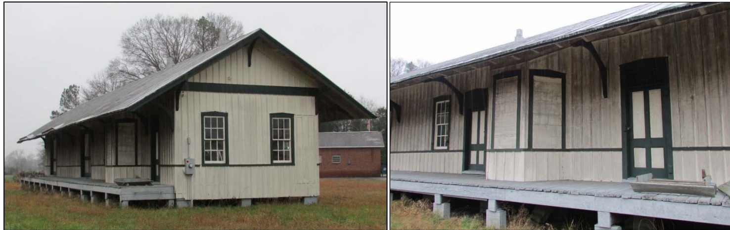
FIGURE 3-81: NORTH OBLIQUE (LEFT); DETAIL OF PROJECTING BAY WINDOW AND DOOR TO PASSENGER WAITING ROOM, EAST ELEVATION (RIGHT)
