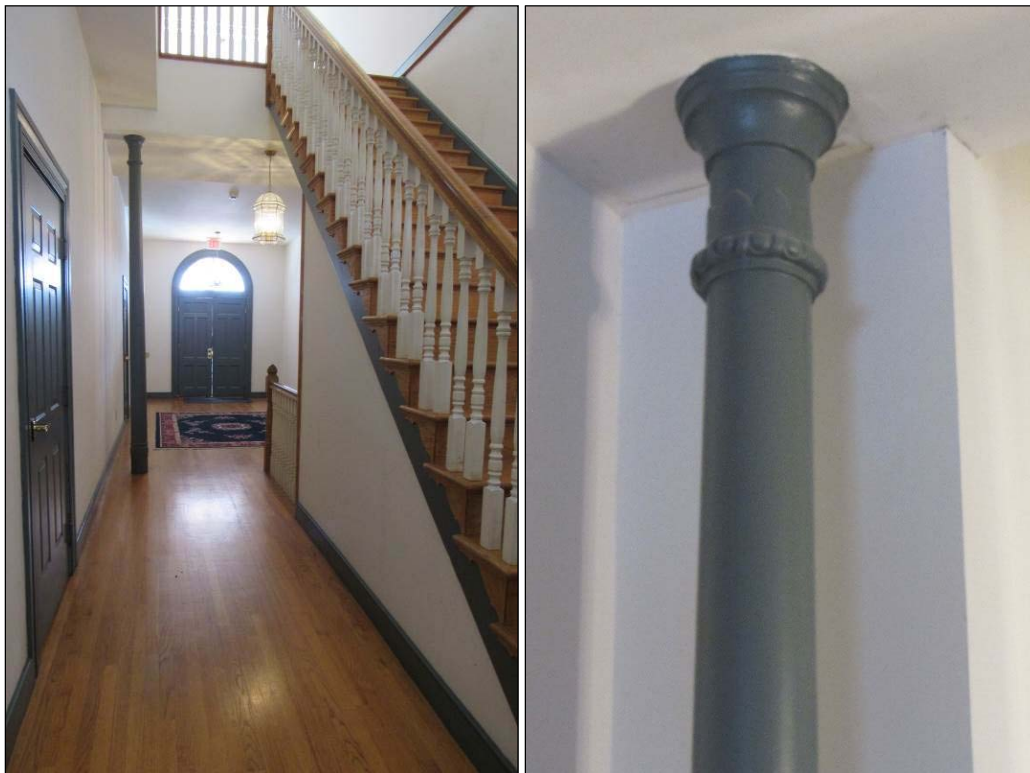
FIGURE 3-216: VIEW OF FIRST STORY HALL, LOOKING EAST (LEFT); DETAIL OF FIRST STORY METAL SUPPORT (RIGHT)
