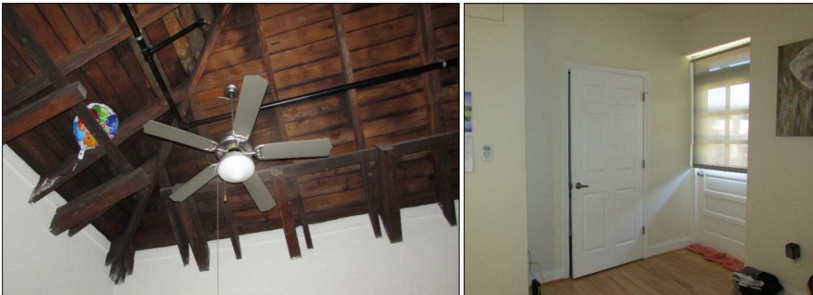
FIGURE 3-257: EXPOSED ROOFING SYSTEM IN THIRD-STORY LOFT (LEFT); VIEW OF “ROMEO AND JULIET” DOOR IN THIRD-STORY LOFT, LOOKING WEST (RIGHT)
