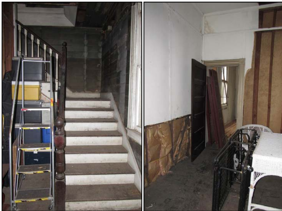
FIGURE 3-189: STAIRWELL LEADING TO SECOND STORY, LOOKING SOUTHWEST (LEFT); FIRST STORY BEDROOM, LOOKING SOUTH (RIGHT)
