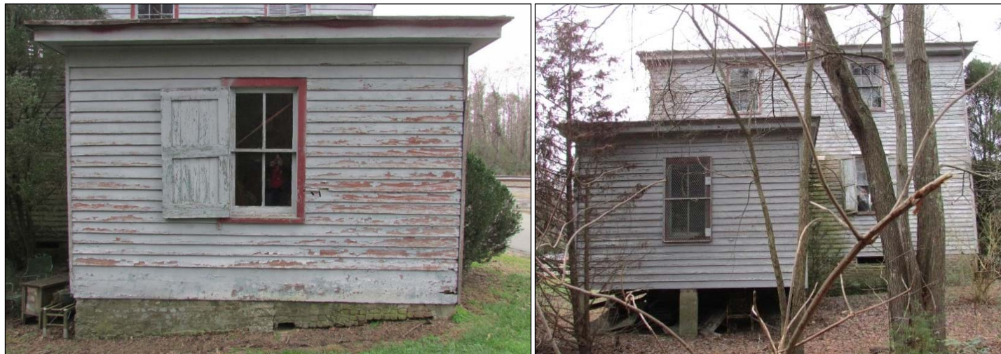
FIGURE 3-141: STORE, DETAIL OF NORTHWEST ADDITION, SHOWING BRICK FOUNDATION (LEFT) AND NORTHEAST ELEVATION OF CENTRAL BLOCK AND NORTHEAST ADDITION (RIGHT)
