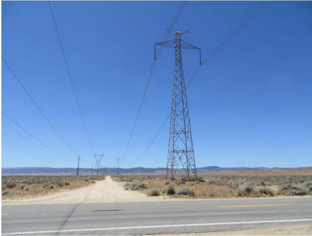
LADWP Transmission Line, view towards the south
