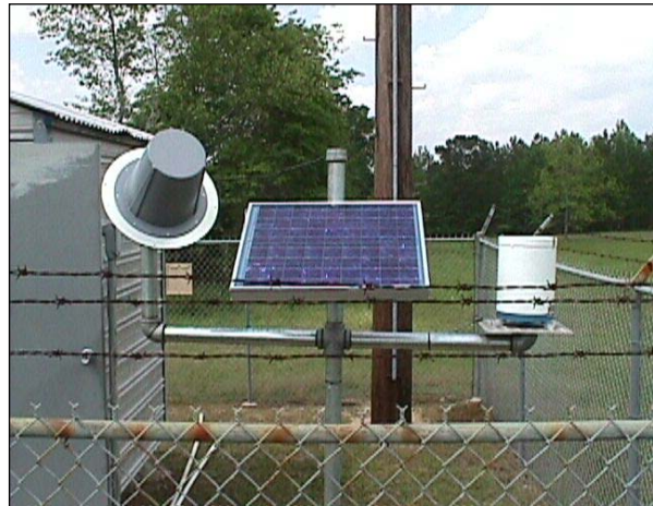
Figure 5-2. Typical Field Installation of a Precipitation Gage
