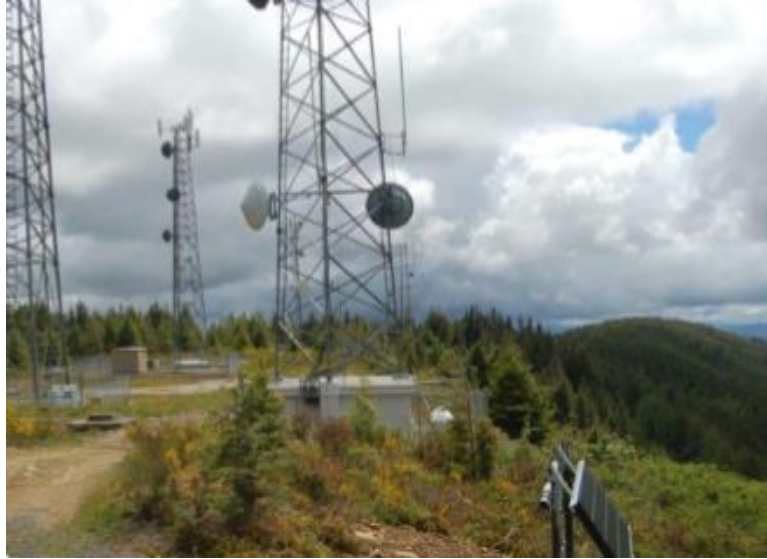
The Radar Ridge communication site in Pacific County (South Coast planning unit). Photo: DNR
