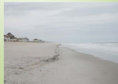
Wet beach with scarp formed on Figure Eight Island (March 18, 2008)
