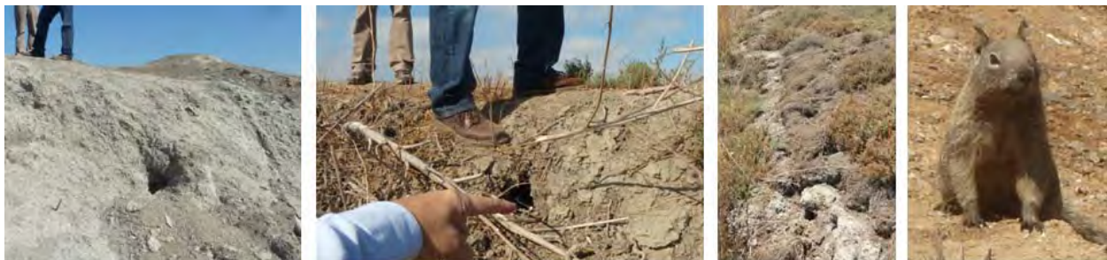
Figure 11 - Rodent dug tunnels are throughout the dike system
