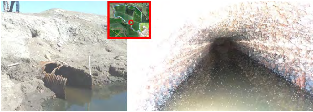
Figure 18 - Pipes through the dike are likely having rusting issues
