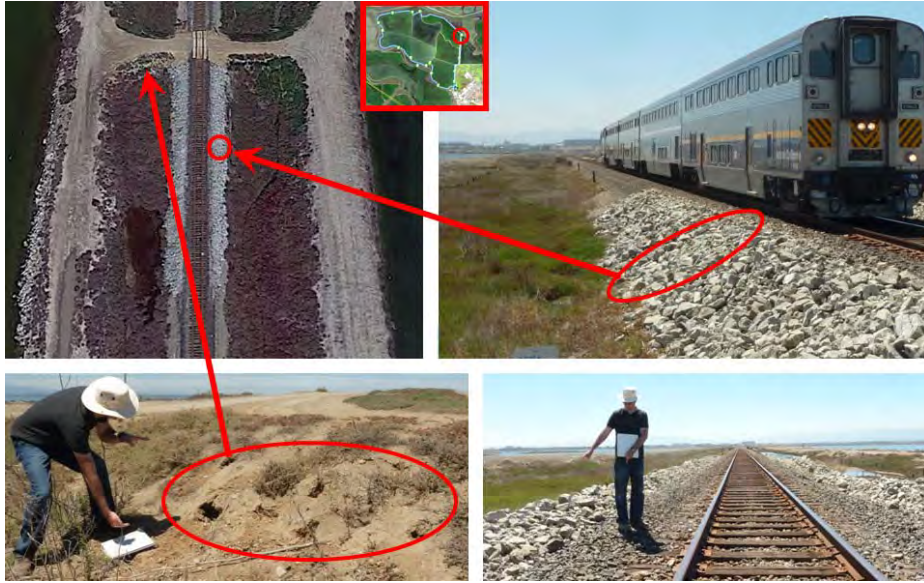
Figure 12 - Rodent dug holes next to railroad crossing
