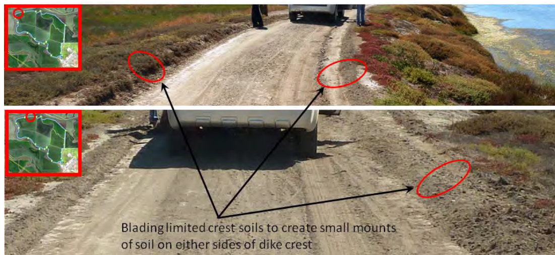
Figure 6 – Blading and scarifying dike crest silt to either side of the crest – to create limited crest elevation rise.
