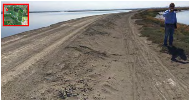
Figure 5 - Loose silt like behavior on dike crest
