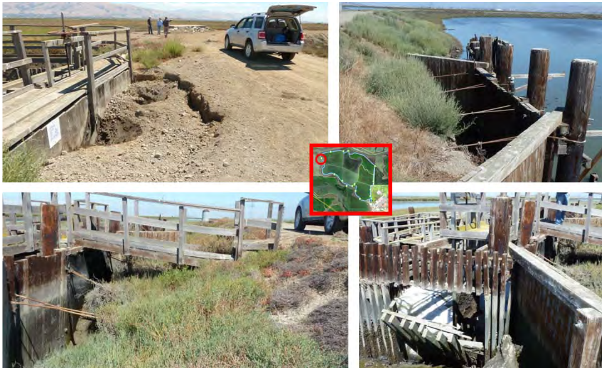
Figure 17 - Water Control structures are experiencing lose of soil issues
