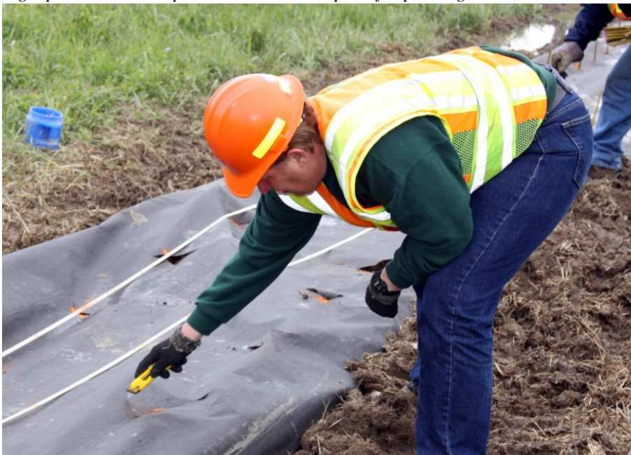
Barb Balcerzak, from Erie South Residency, is cutting the landscape cloth with an "x" pattern in advance of planting the willows.
