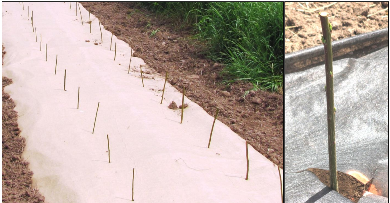
Figure 3 (left) – Willow cuttings installed through paper landscape fabric in a double row pattern Figure 4 (right) – Willow cuttings planted to the proper depth with the buds facing upwards Photos by SUNY ESF
