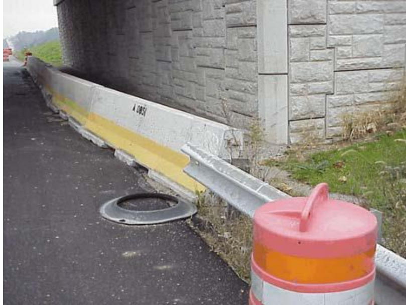
Figure 1. Unsafe Connection between Guardrail and Portable Concrete Barriers
