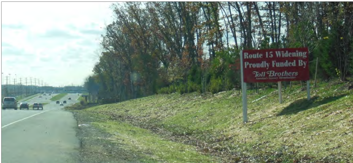
Figure 9. Sign Along U.S. 15 in Prince William County Notes Homebuilder's Participation in Road Widening Costs
