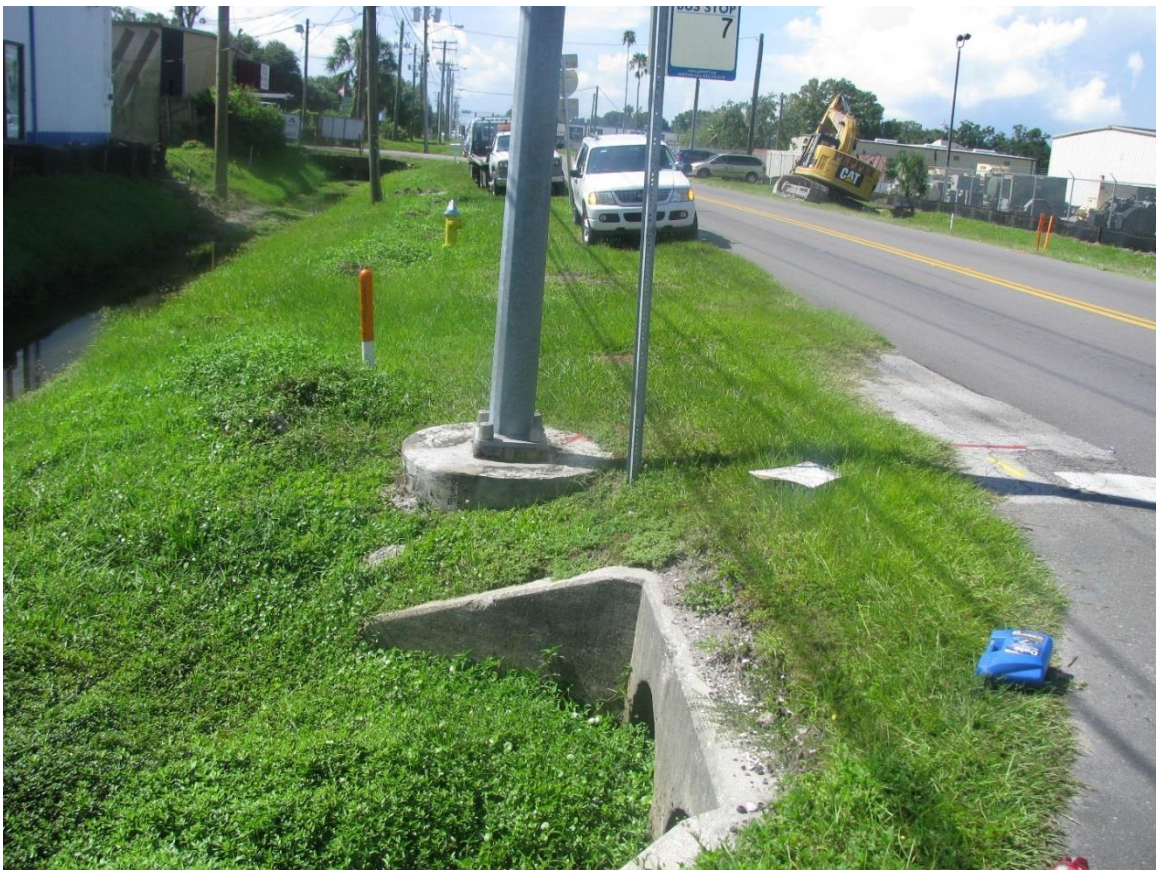
Figure 5-20: Bus Stop Close to Drainage
