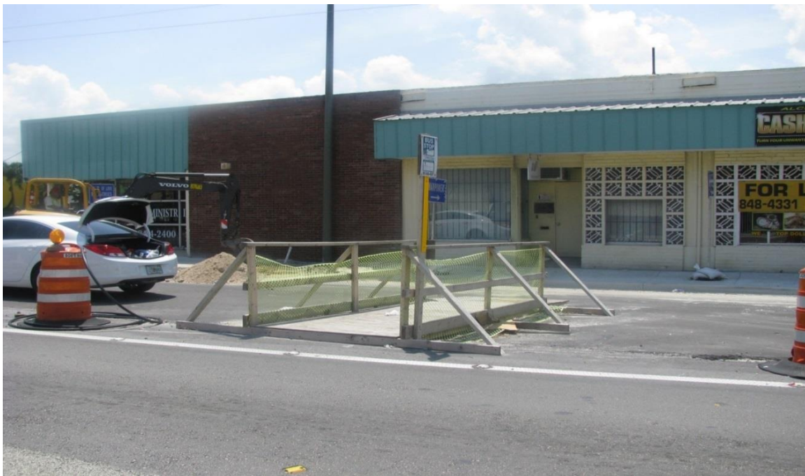
Figure 5-16: Non-Compliant Pedestrian Platform
