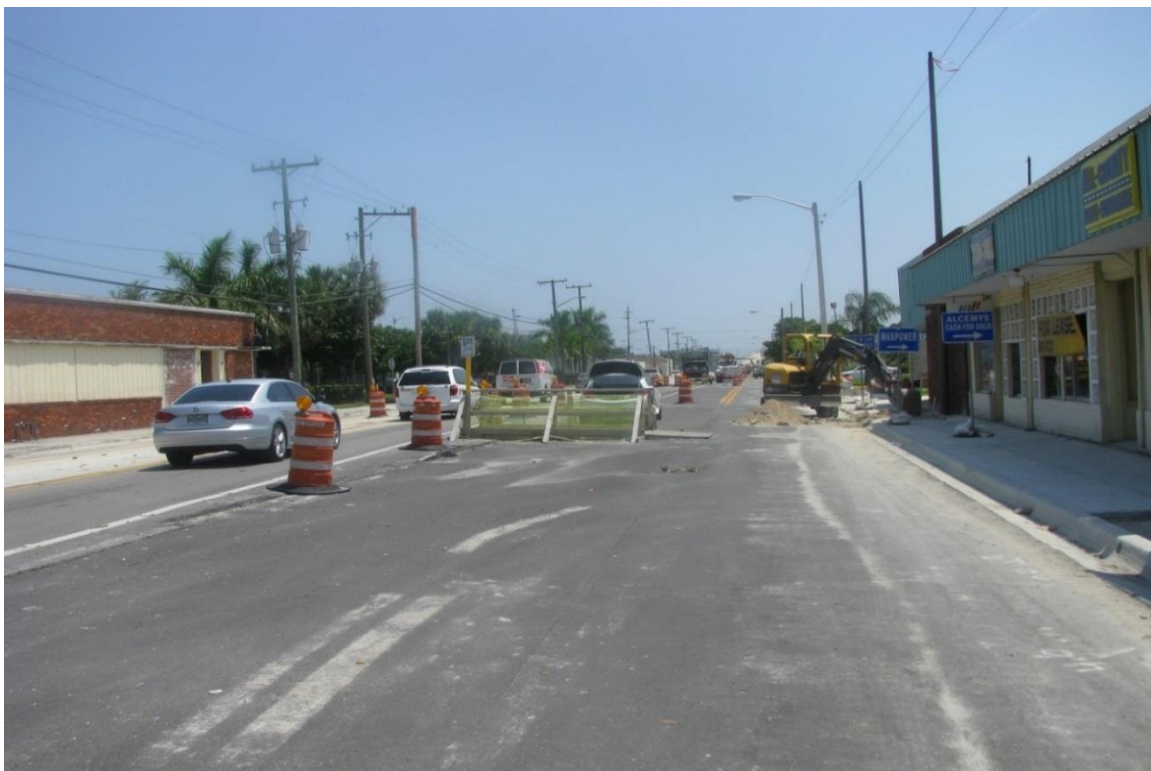
Figure 5-17: Inadequate Bus Stop Access
