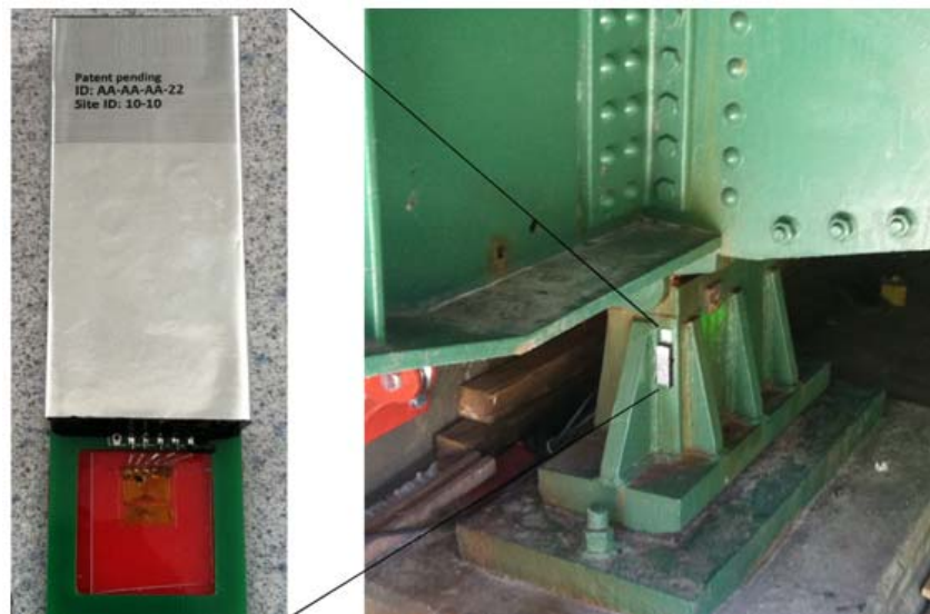
Figure 1: A SenSpot (left) and installed sensor on a bridge bearing (right) for tilt and loading monitoring.
