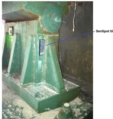
Figure 8: Wireless tilt sensor on a rocker bearing of Northwest Branch Bridge on I-495
