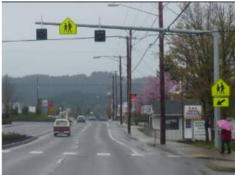
Figure 5.3: Overhead beacon installation in Philomath, Oregon
