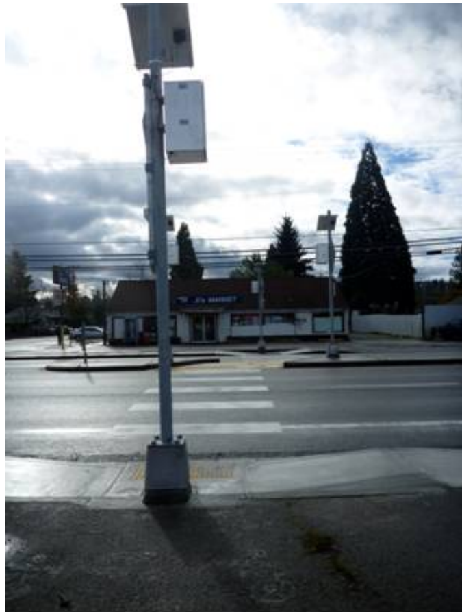
Figure 5.9: Pedestrian perspective of RRFB installation on Main Street in Springfield
