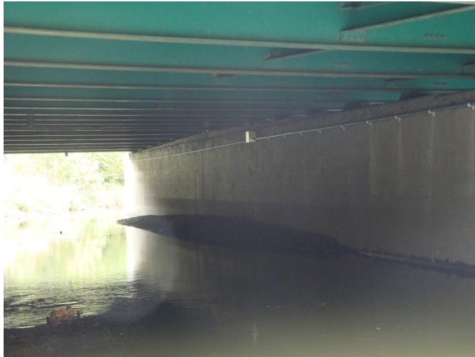
Figure 7. Accumulation of sediments along the abutment wall due to upstream scour.
