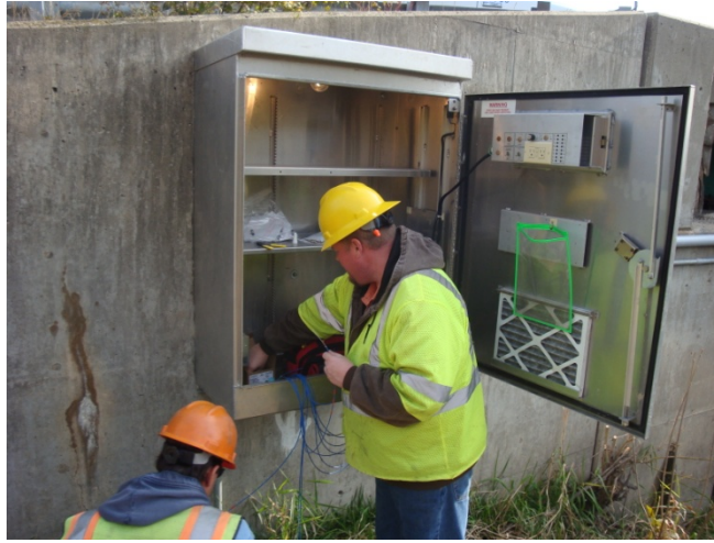
Figure 9. Nema enclosure box to house the instrumentation.
