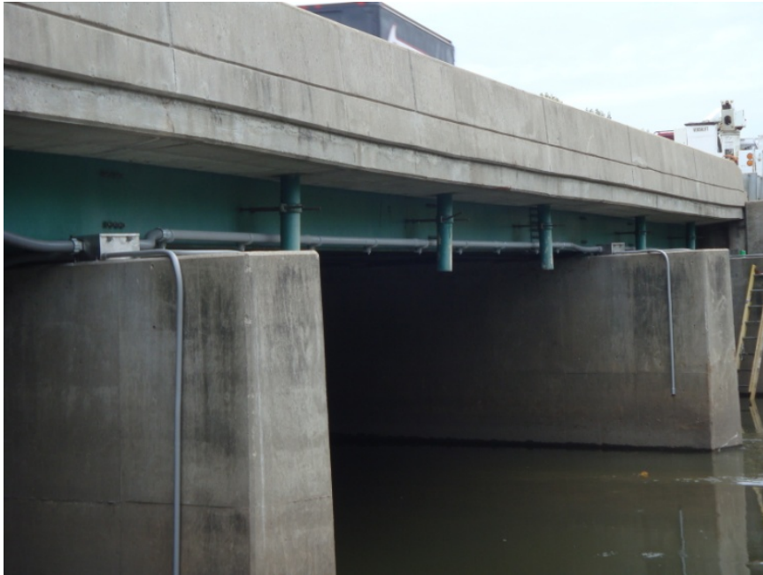
Figure 10. Typical junction boxes on the bridge piers with conduit lines to sensors.
