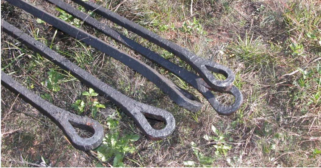
Figure 16. Forge welded loop eyebars from the City of Griffin 6 th St. Bridge.
