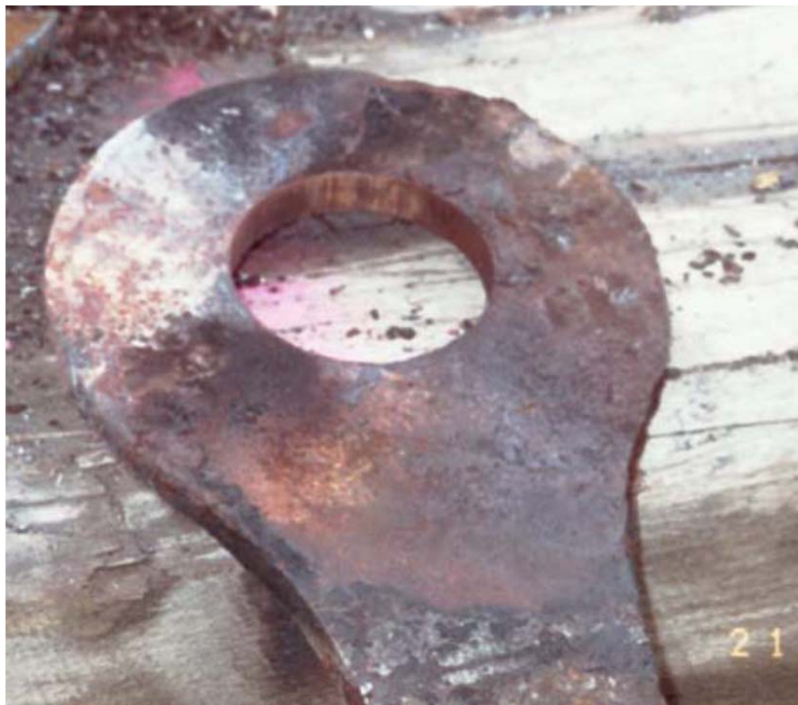
Figure 12. Eyebar end connection showing heavy corrosion (Bowman and Piskorowski 2004)
