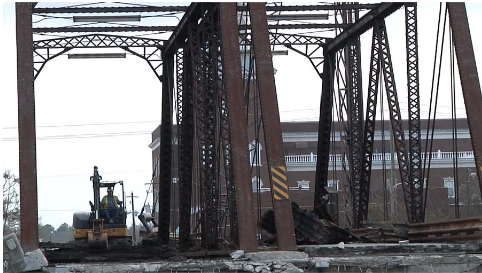
Figure 49. Removal of concrete roadway and timber stringers (Courtesy of Sharman Southall, GDOT).
