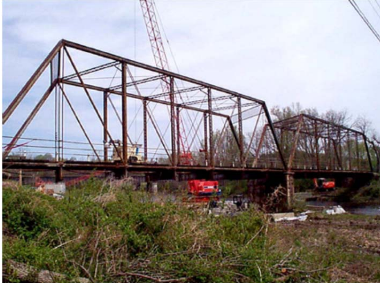
Figure 30. Goshen Bridge, Route 746 Bridge over the Calfpasture River at Goshen, Virginia (VDOT 2006) prior to disassembly.
