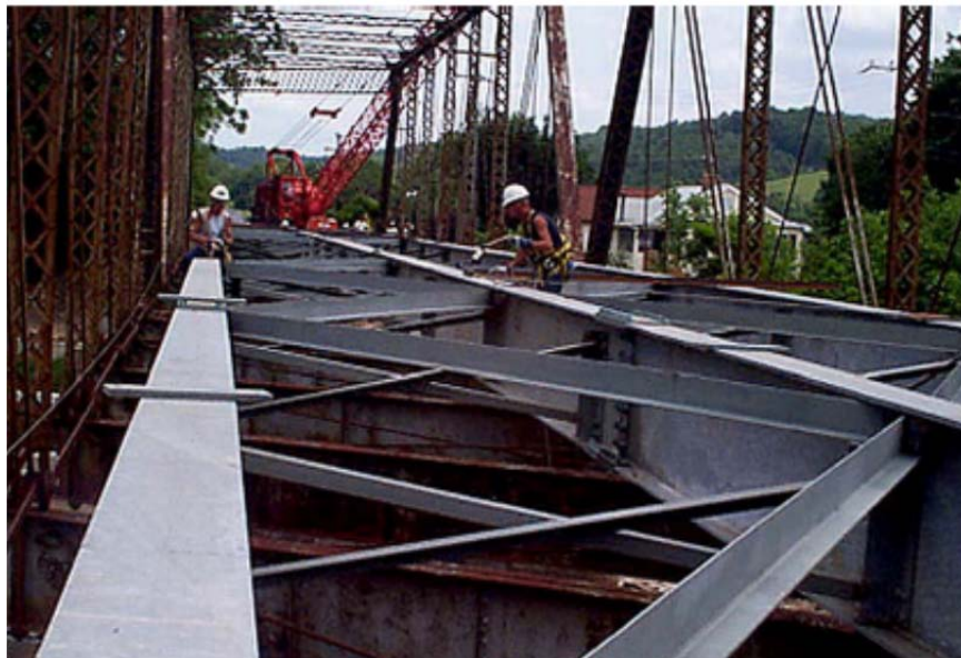
Figure 31. Installation of the beams for the internal two-span continuous falsework bridge used for the disassembly of the Goshen Bridge (VDOT 2006).
