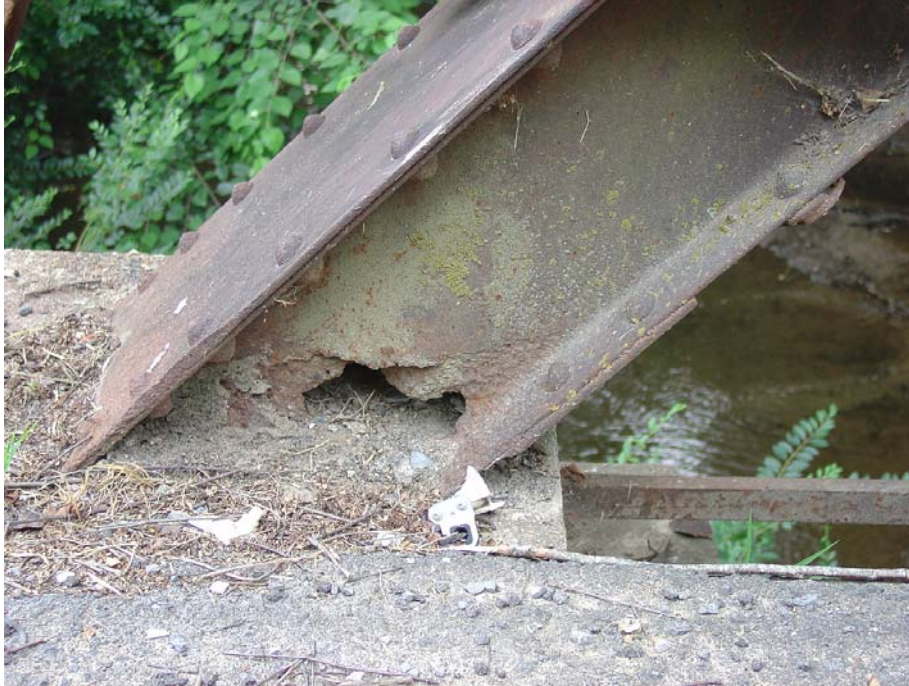
(c) End post detail at the bridge abutment showing some loss of the cross-section due to corrosion
