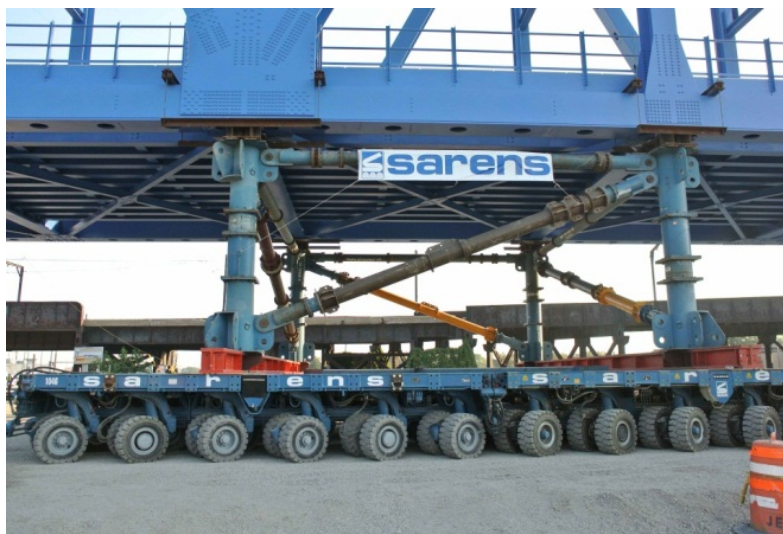
Figure 35. A SPMT moving the Torrence Avenue truss bridge into its erection site in Chicago, Illinois (Transportation Nation 2012).
