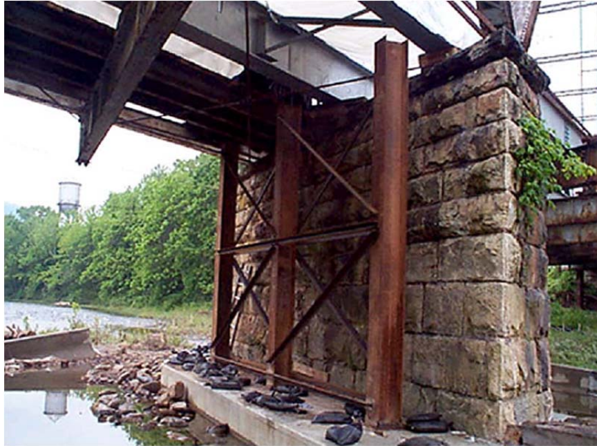
Figure 32. Temporary bent at the middle pier of the Goshen Bridge, with two lines of the falsework beams in place, from (VDOT 2006).
