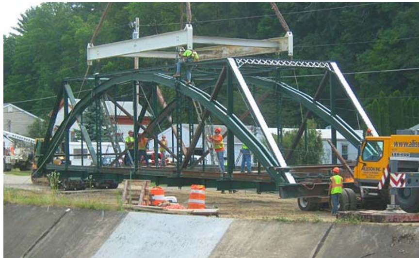
Figure 23. Relocation of the 7th Street Bridge in Coudersport, Pennsylvania (Larson Design Group 2011).
