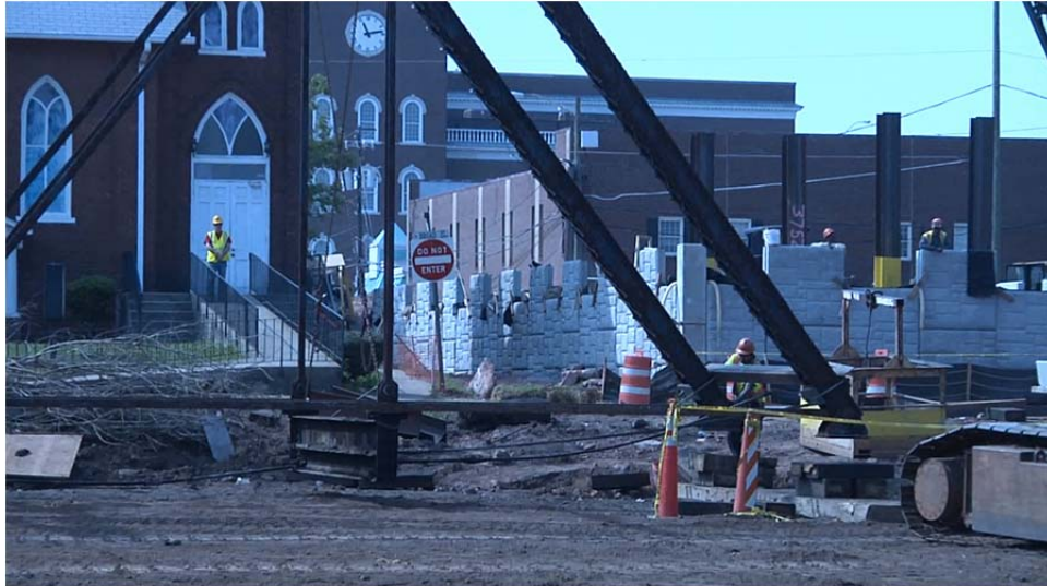
Figure 52. Trusses placed on cribbing at each of the four corner supports to ensure that the five truss verticals remained elevated (Courtesy of Sharman Southall, GDOT).
