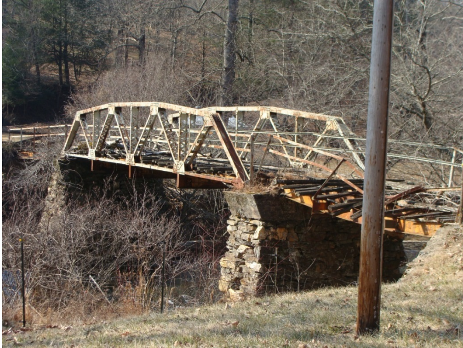
Figure 8. Pony Warren truss located in Fannin County, Bridge 111-9992 in the GHBS (GDOT 2012).
