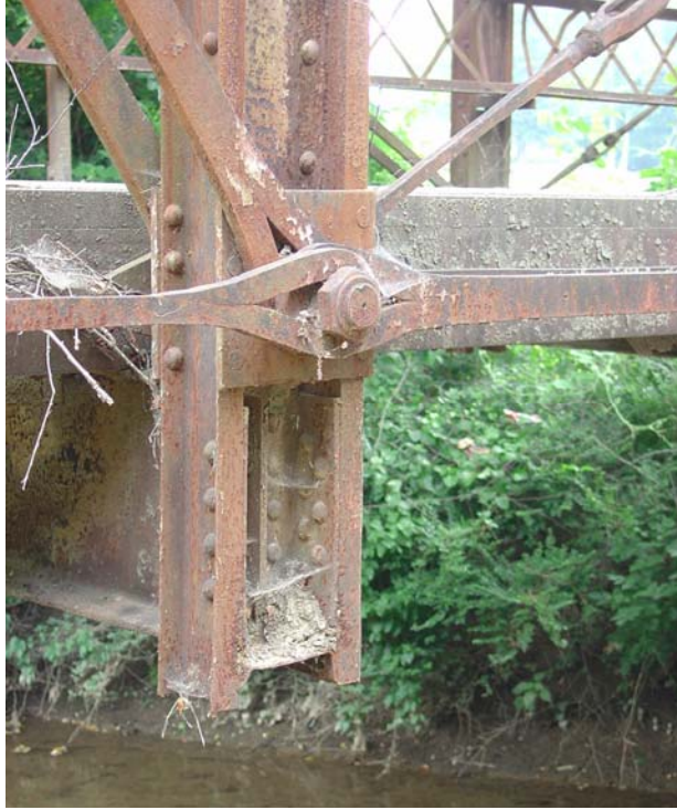
(a) Pin and eyebar member detail at a bottom chord joint, with a floor beam framed into the truss vertical member at the joint.
