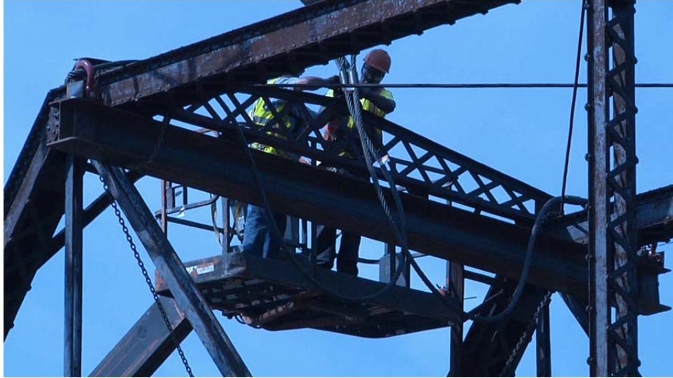
Figure 50. Lateral and horizontal bracing at the upper chord to accommodate the crane lift points (Courtesy of Sharman Southall, GDOT).
