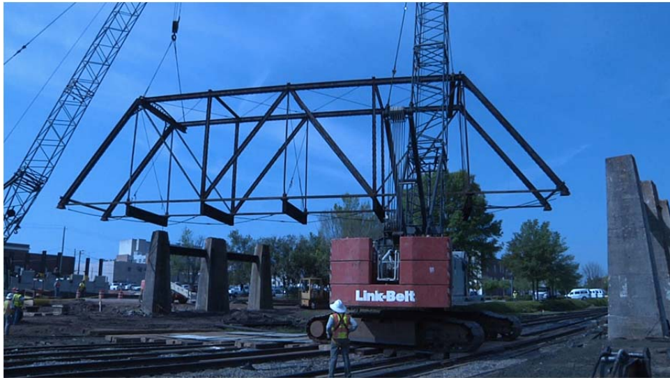
Figure 51. Two cranes working together to lift the 100 feet span (Courtesy of Sharman Southall, GDOT).
