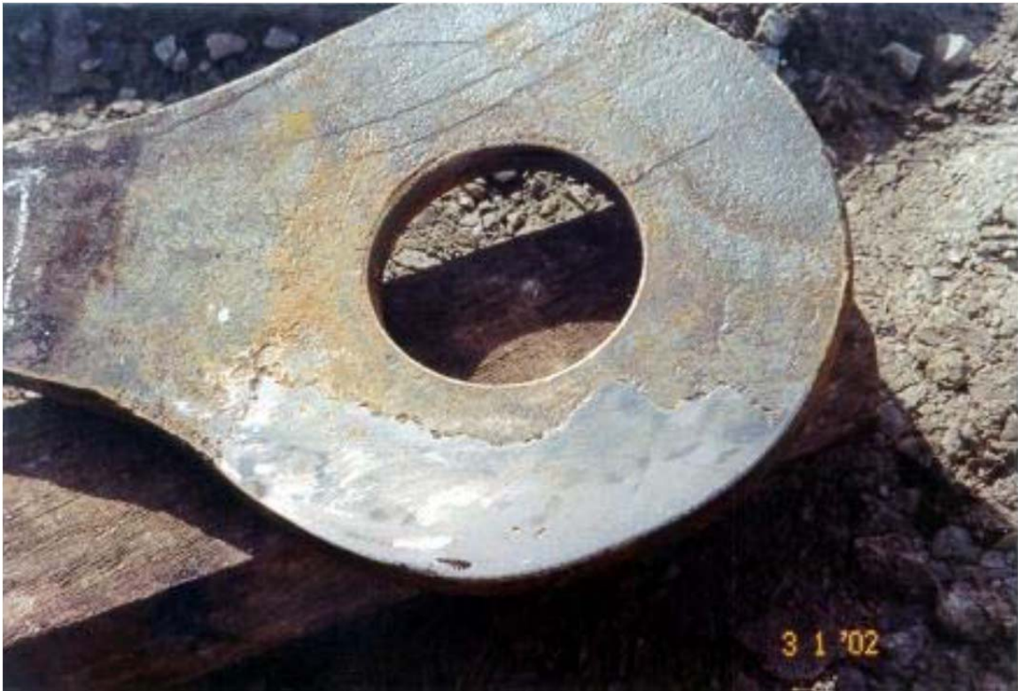
Figure 13. Eyebar end connection after repair by the filler weld procedure (Bowman and Piskorowski 2004)
