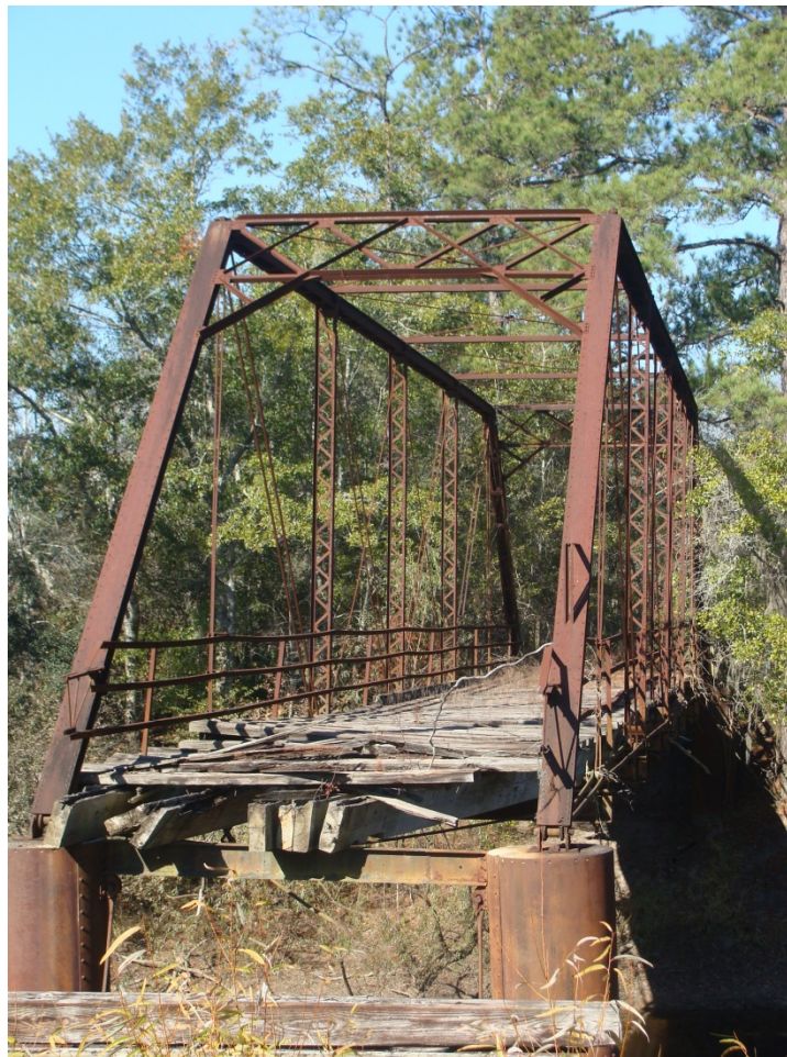
Figure 5. One-hundred ft. span Pratt (pinned) thru truss located in Thomas County, Bridge 275-9991 (GDOT 2012).
